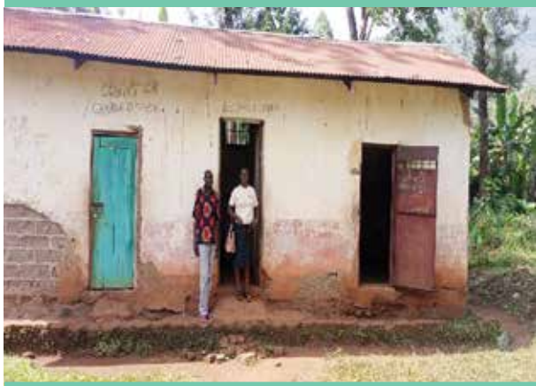
Dilapidated offices and cells of Bukigai Police Post in Bududa District
