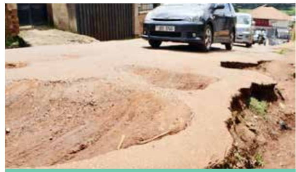
A pothole on one of the roads in Kampala
