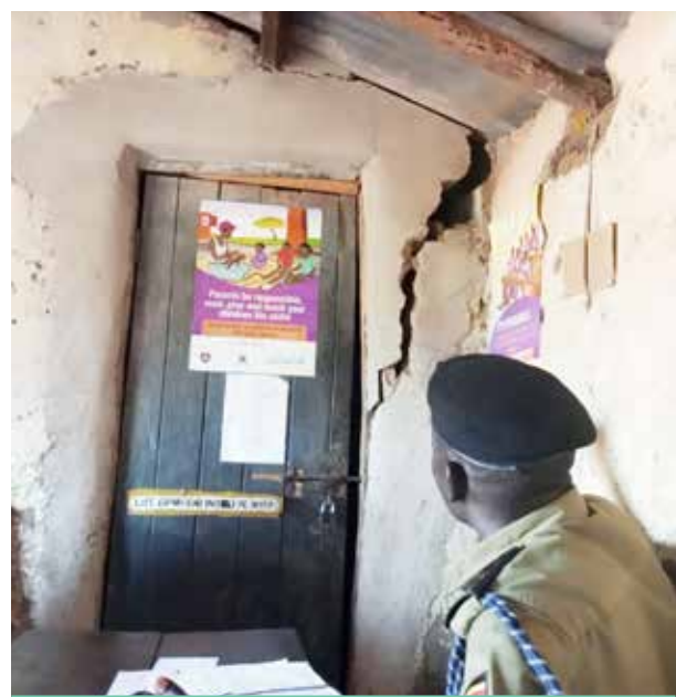
Dilapidated Akia Police Post in Lira City with a cracked interior wall
