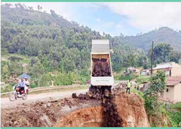
UHRC official inspecting road repairs along a section of Kabale-Kisoro Road which had been washed off by heavy rains.
