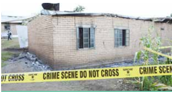
One of the dormitories burnt by the ADF during the attack at Mpondwe Lhubiriha Secondary School.
